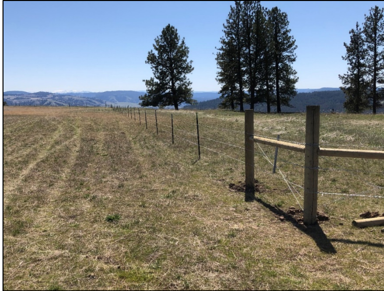
Completed interior drift fence at the Airport fields on the west permit area
