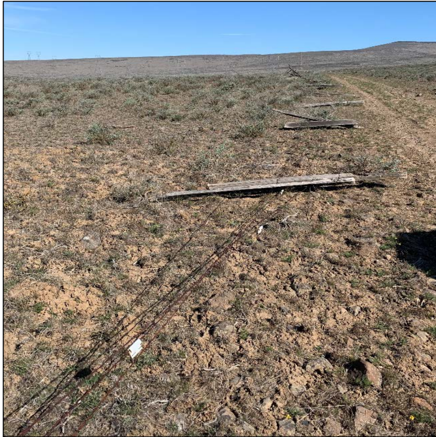
A small sample of fencing in need of repair in the Quilomene Wildlife Area
