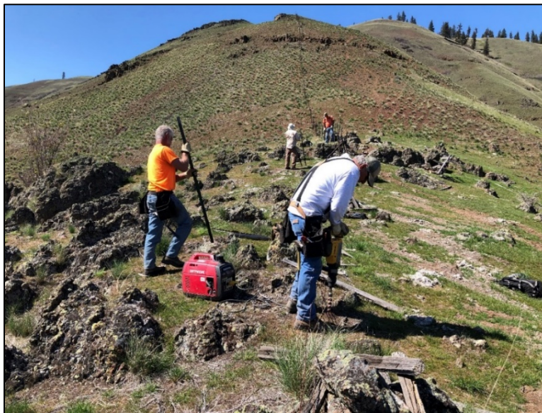
Dave Meisner drills a hole in the rock for a t-post while Scott McGee, David Woodall, and Greg Heimgartner are hard at work!
