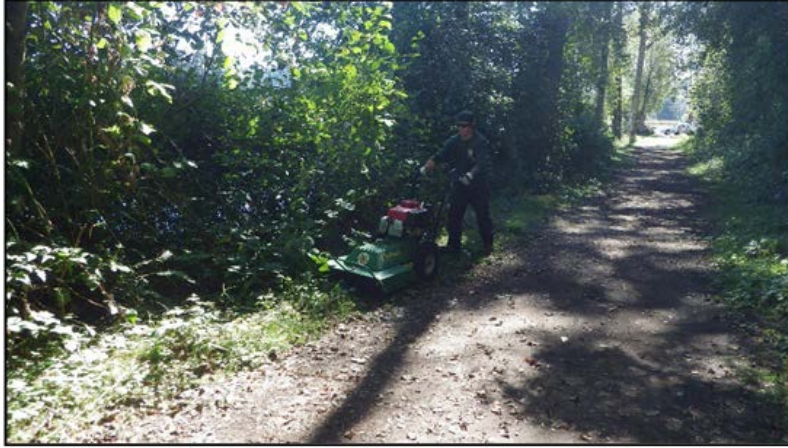
Access staff member Holt using walk behind brush cutter at the Kress lake trail to clear brush
