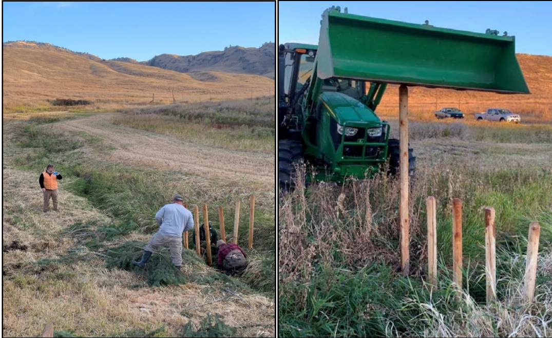
Soft ground allowed us to push the poles in place. Archeologist Kelly monitoring the installation and staff members weaving fir boughs into the log structure. - Photos by Olson
