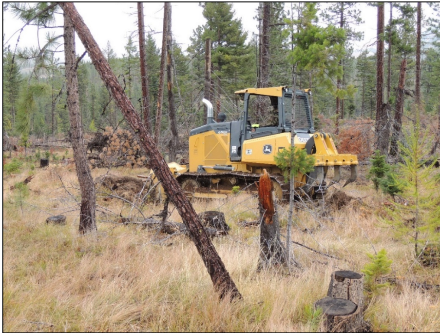
Dozer working to develop firelines in Stemilt Basin on the Colockum Wildlife Area
