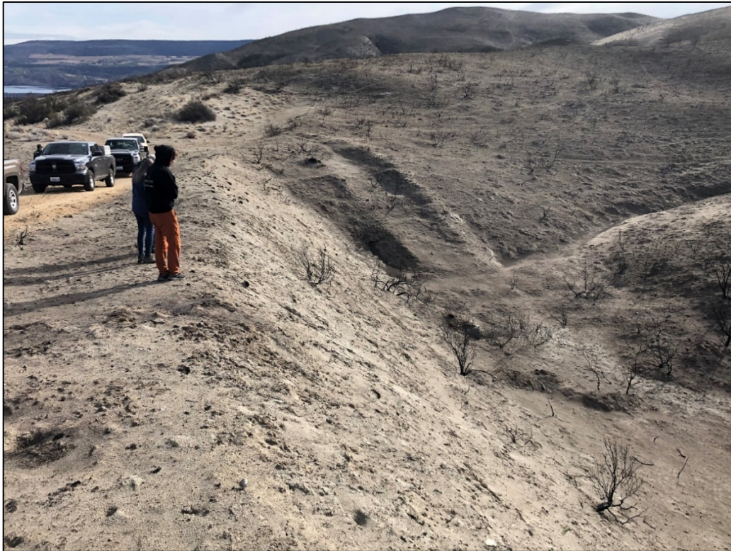
Assessing and discussing next steps to reduce likelihood of culvert blockages from runoff and debris flows - Photo by Finger
