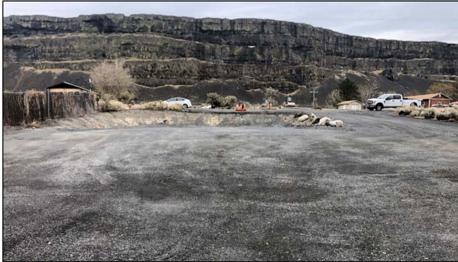
Blue Lake Water Access Site looking inland from the start of the plank launch, paving will be completed by the end of October - Photo by Finger
