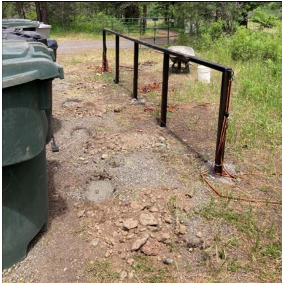
Anchor points set in concrete to secure garbage containers at a remote summer camp location in Columbia County
