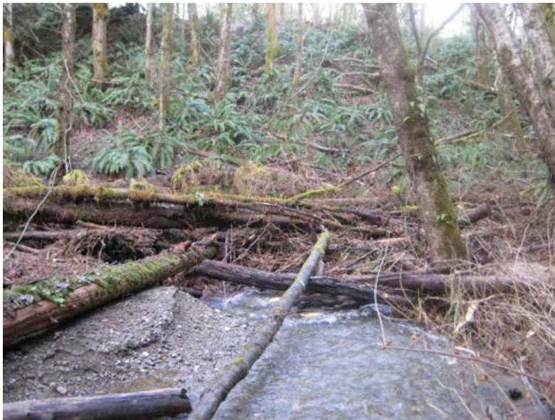
Photos of Dickerson Creek at the Navy railroad, view looking downstream. Upper photo from October, 2012 (photo by Tim Abbe, NSD). Lower photo from December 2010 shows blockage of the 48" diameter culverts (photo by Jon Oleyar, Suquamish Tribe).
