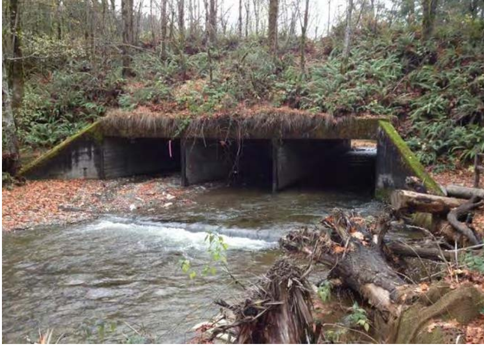
Photo of the triple box culvert at NW Golf Club Hill Road (view upstream). Photo taken November 2012 by Shawn Higgins, NSD.
