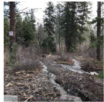
2-9-20 Washed-out Asphalt South of Campground 4
