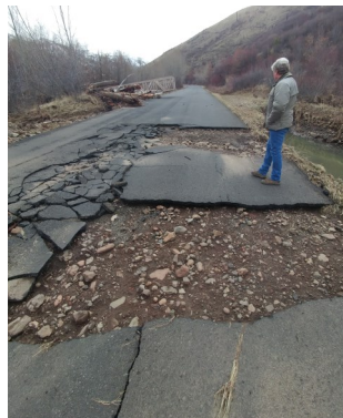
2-9-20 Washed-out Asphalt South of Campground 4
