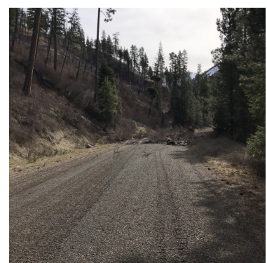
3-10-20 Mudslide just north of Campground 10
