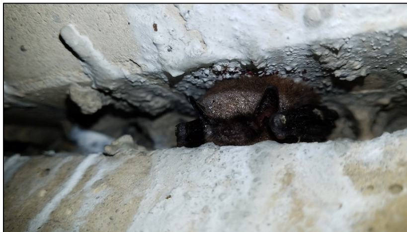
A western long-legged bat ( Myotis volans ) roosting in an expansion gap of a bridge
