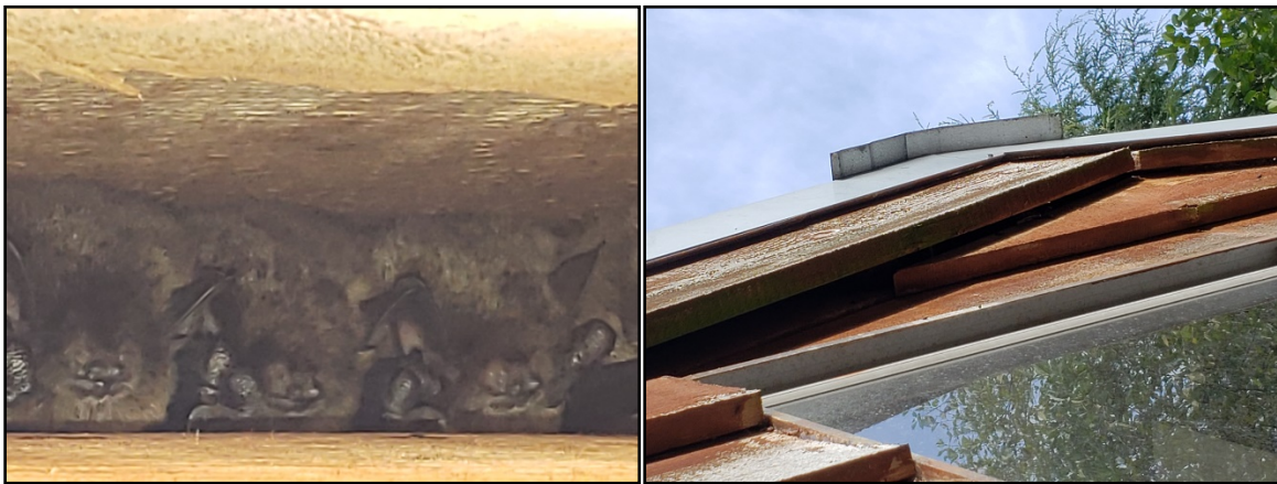
Bats documented roosting between siding boards of greenhouse
