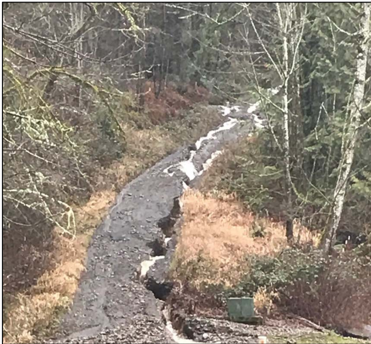
One of several impassable roads recently encountered during East/West Bear Project
