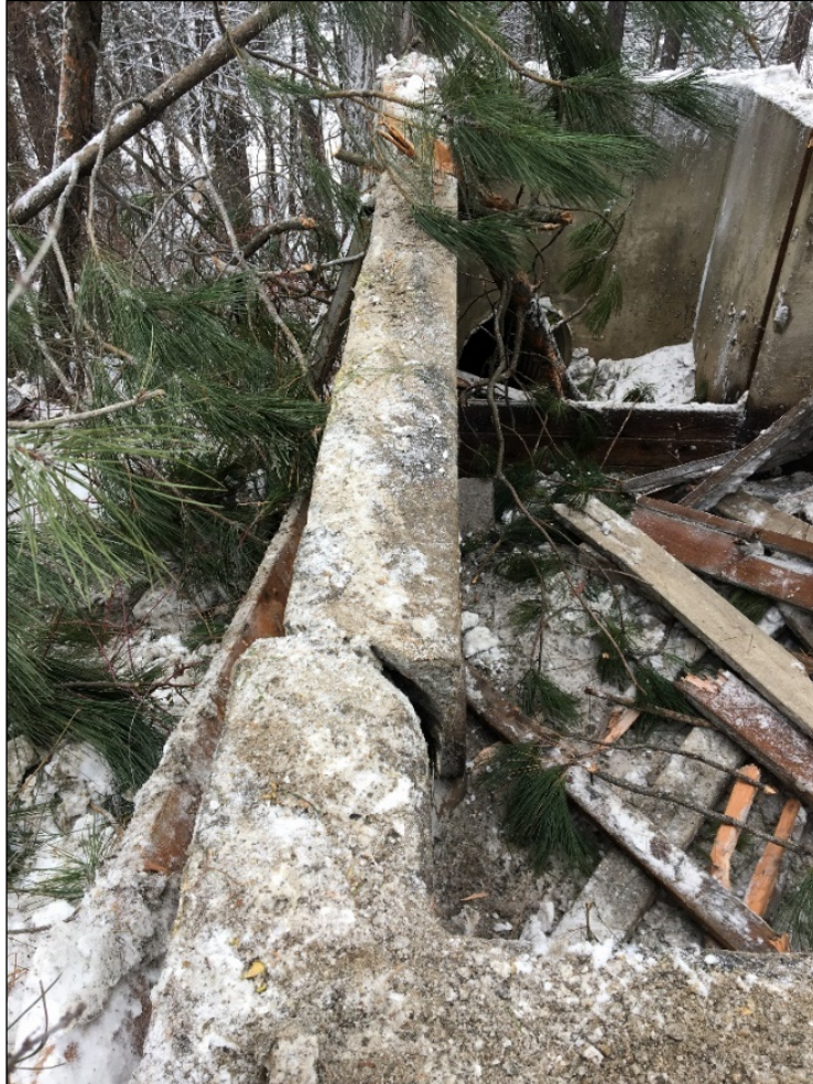
Damaged concrete wall, wooden lid, and dam boards
