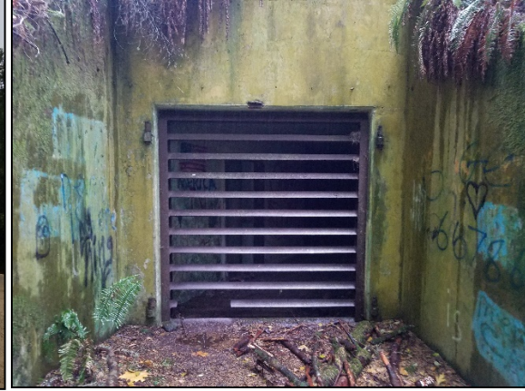
Striped Peak Bunker – vandalism to gate
