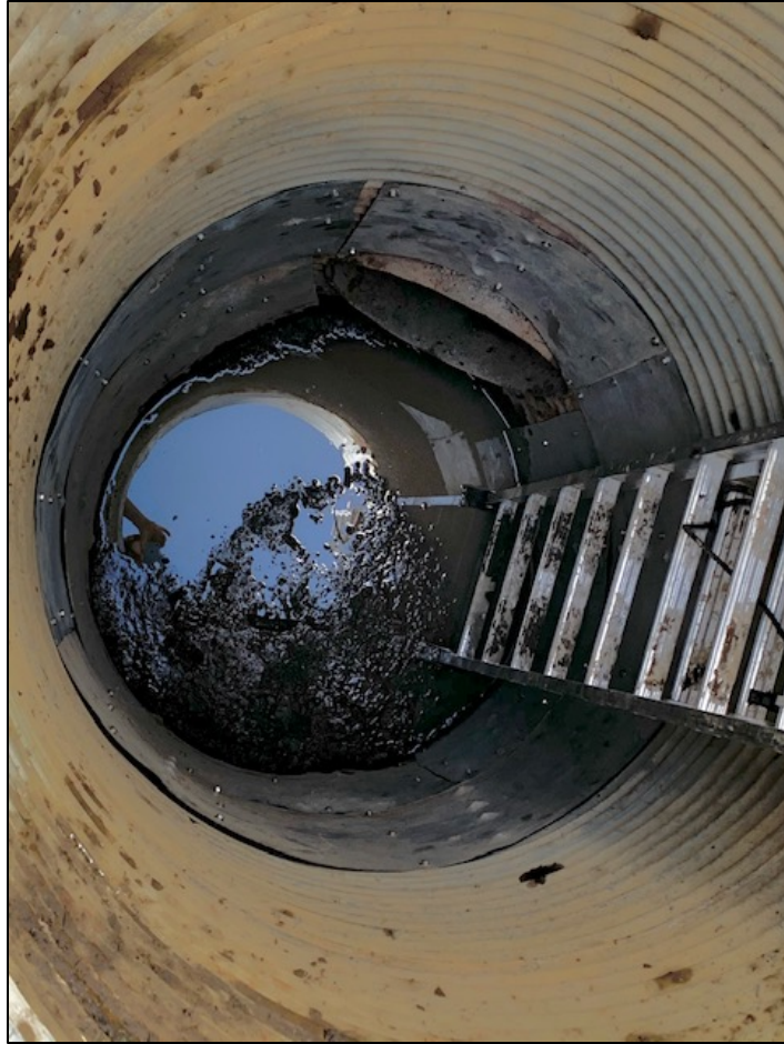
Repaired section of lift pump structure showing new steel lining over corroded areas
