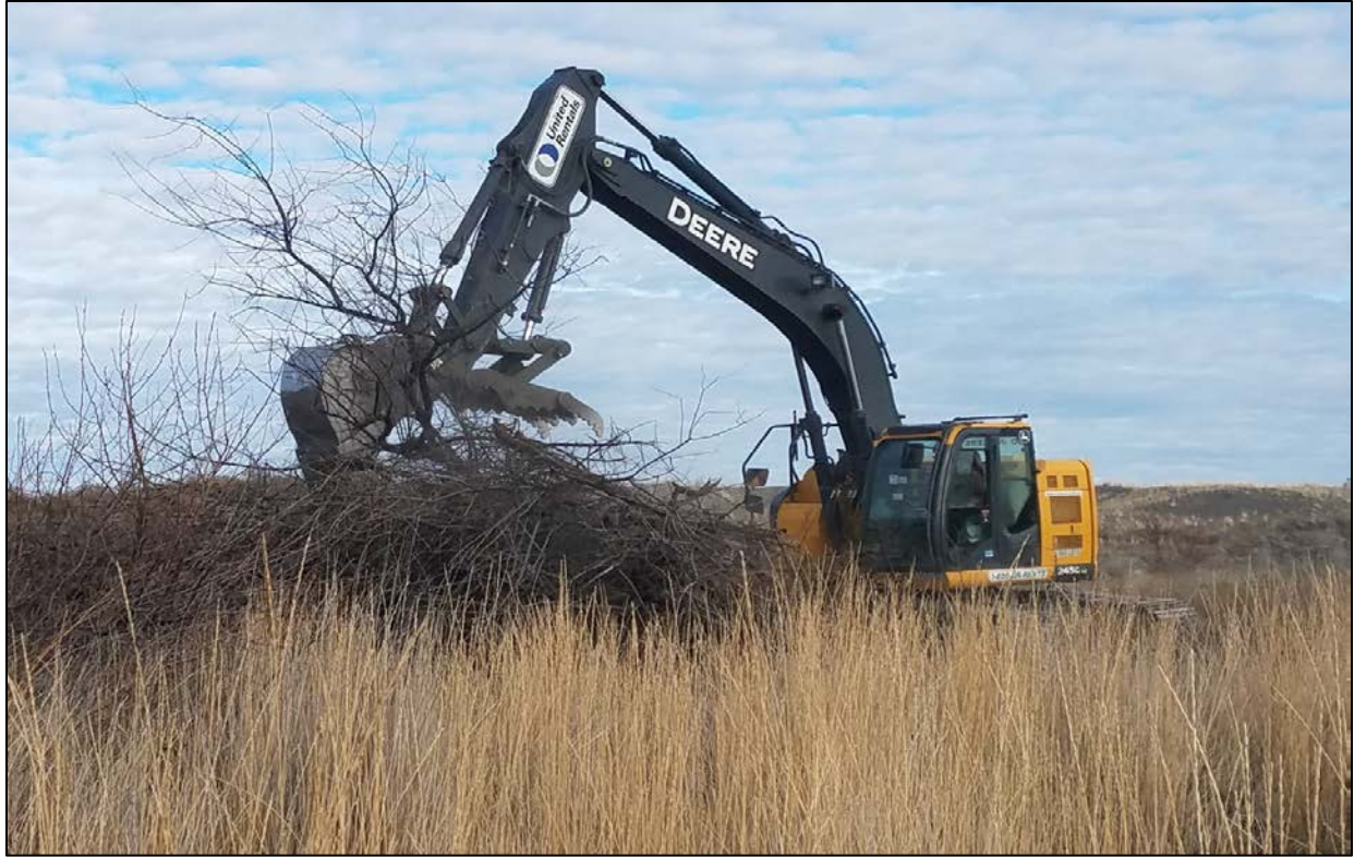
Russian olive removal work in the expansion – Photo by C. McPherson and B. Cole
