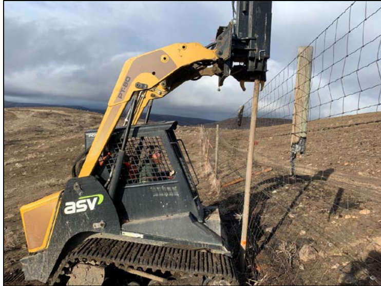
Natural Resources Technician Stultz driving metal sucker pipe along burnt section of the Bull Pasture elk fence
