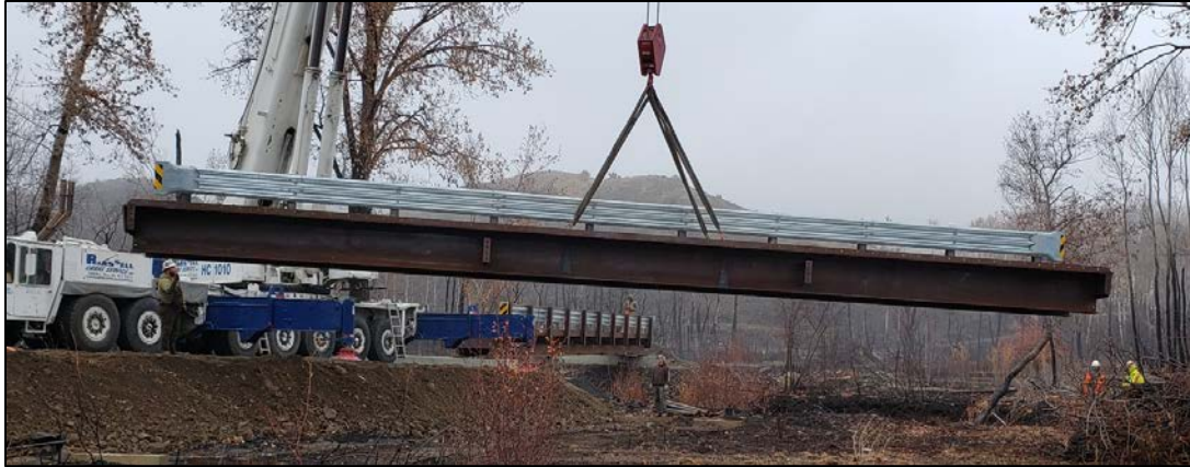
Crane installing second half of new vehicle bridge at Hardy Canyon crossing
