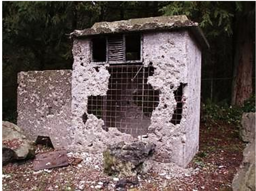
View of the vandalized Lake Tarboo restroom before removal.
