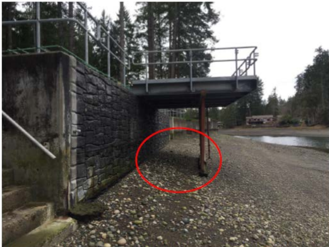
Photo taken by Allison Cook on March 2 nd , 2018. Shows overwater deck, pin piles, and bulkhead replacement. Shading from overwater structure is identified by red circle in the photo.
