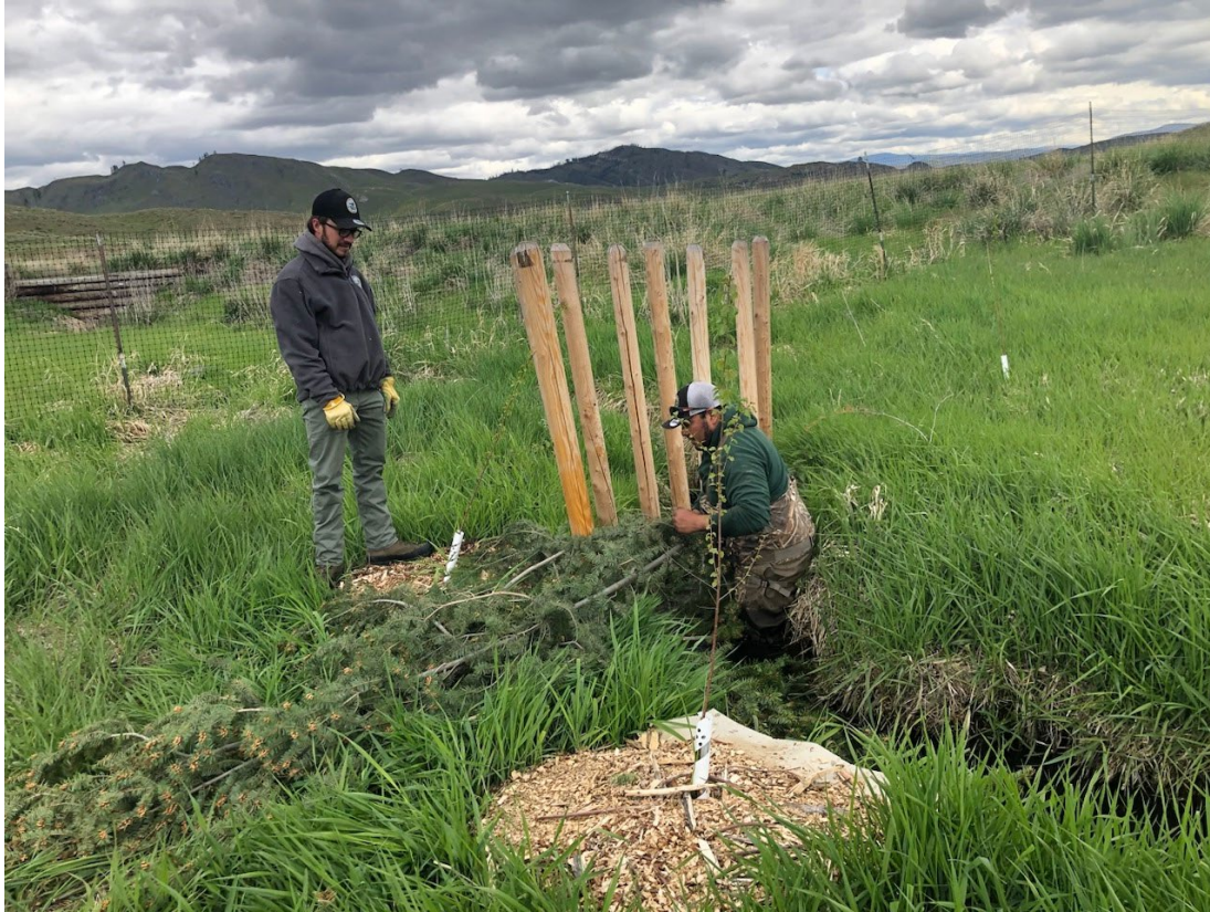
WDFW staff adding fir boughs to a BDA within the project area.
