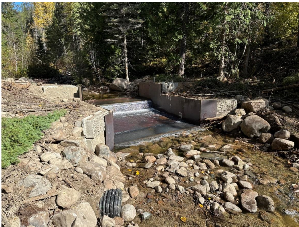
Figure 2. West Branch LeClerc Creek temporary fish management structure.
