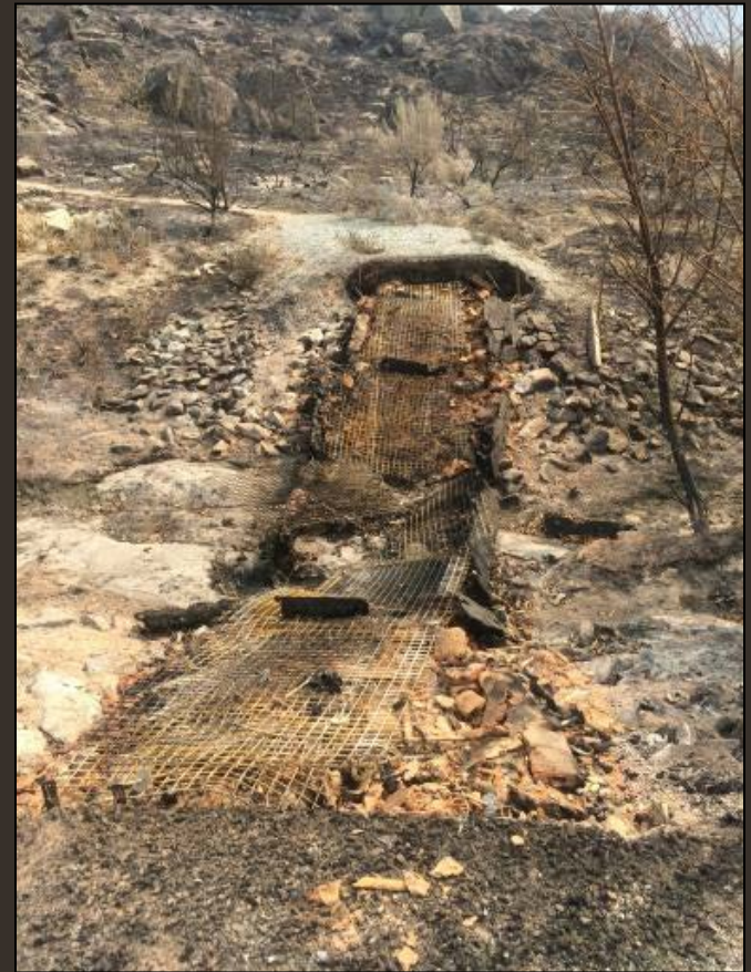
Remains of pedestrian bridge over Toad Creek at Beebe Springs
