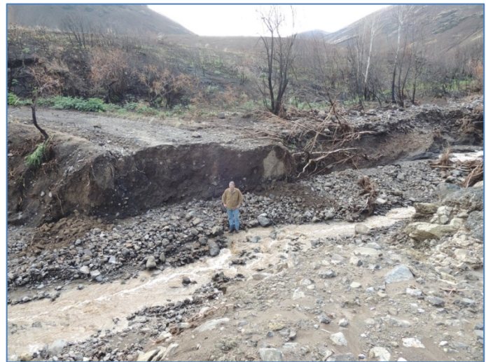
Flood damaged road on Colockum Wildlife Area, Sept. 2013.
