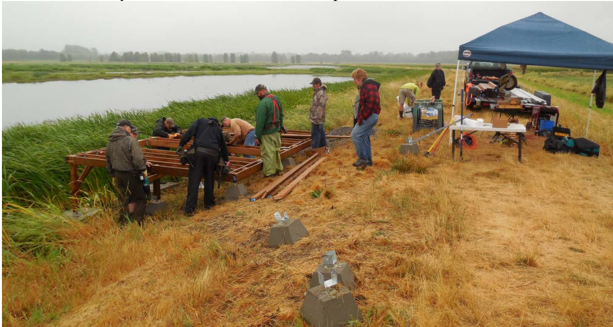
Washington Waterfowl Association work party constructing new ADA blind platform on the South Cell wetland.
