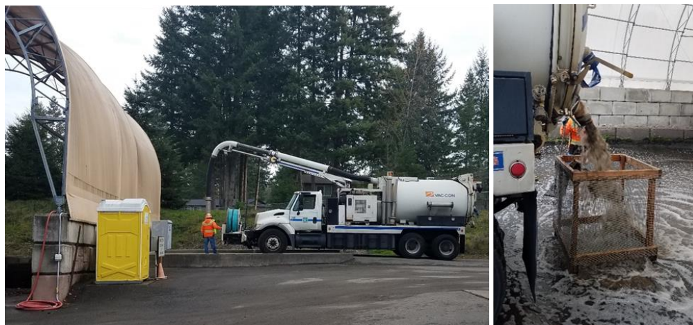
Figure 8. City of Lacey storm sewer vacuum truck transports ACF along with debris during annual maintenance.
