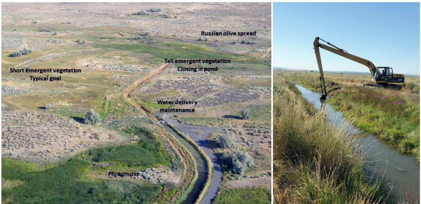
Left: Typical management challenges associated with wildlife area wetlands. Right: Ditch cleanout
