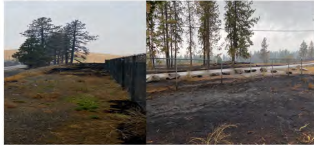
Figures 19 & 20: The structural integrity of burned fencing around utility and boundary areas are no longer safe and must be replaced. Dziekan, Water Access Manager
