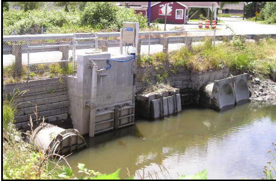
Figure 1-1. Tidegates on Edison Slough, various top-hinged gates and a Self Regulating Tidegate (center left). County maintained tidegate complex.
