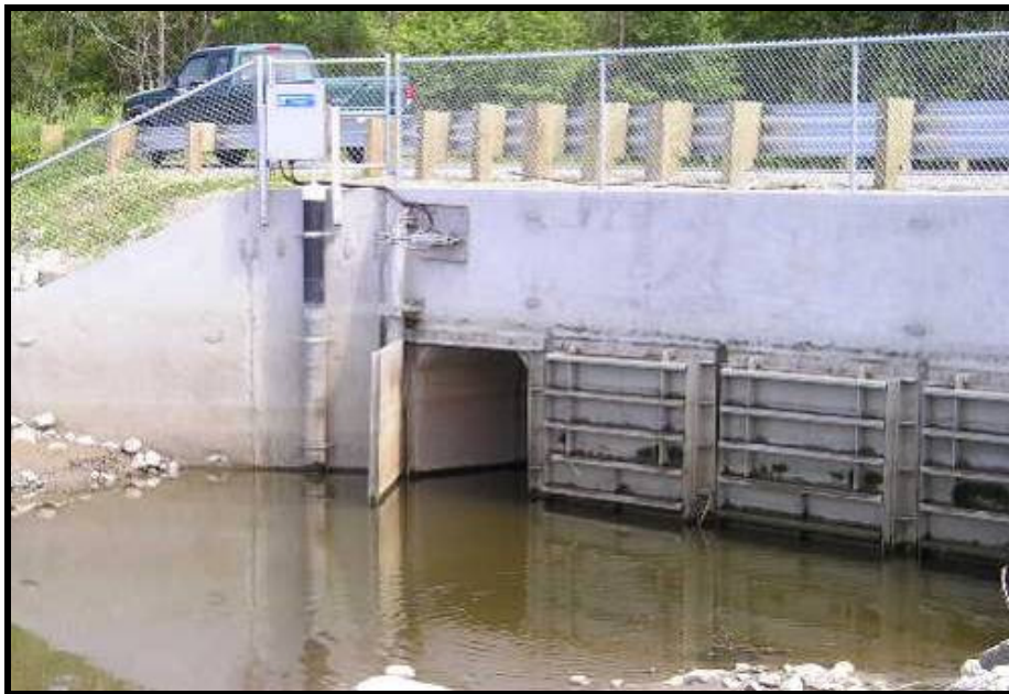
Figure 4-2. McElroy Slough Automatic Regulating Tidegate, “Aberdeen” style gate, open at a -2.7 foot tide event (County owned tidegate complex).
