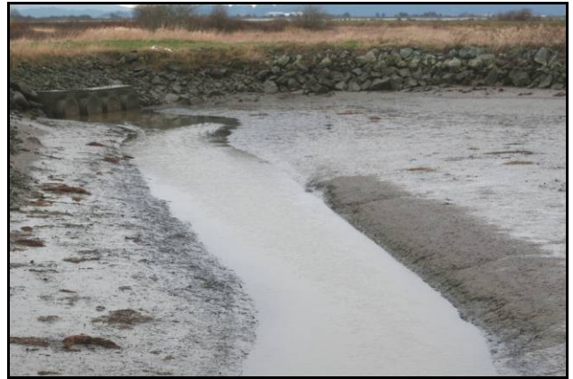
Figure 14. Downstream of Tidegate Complex 35 showing accumulated sediment.
